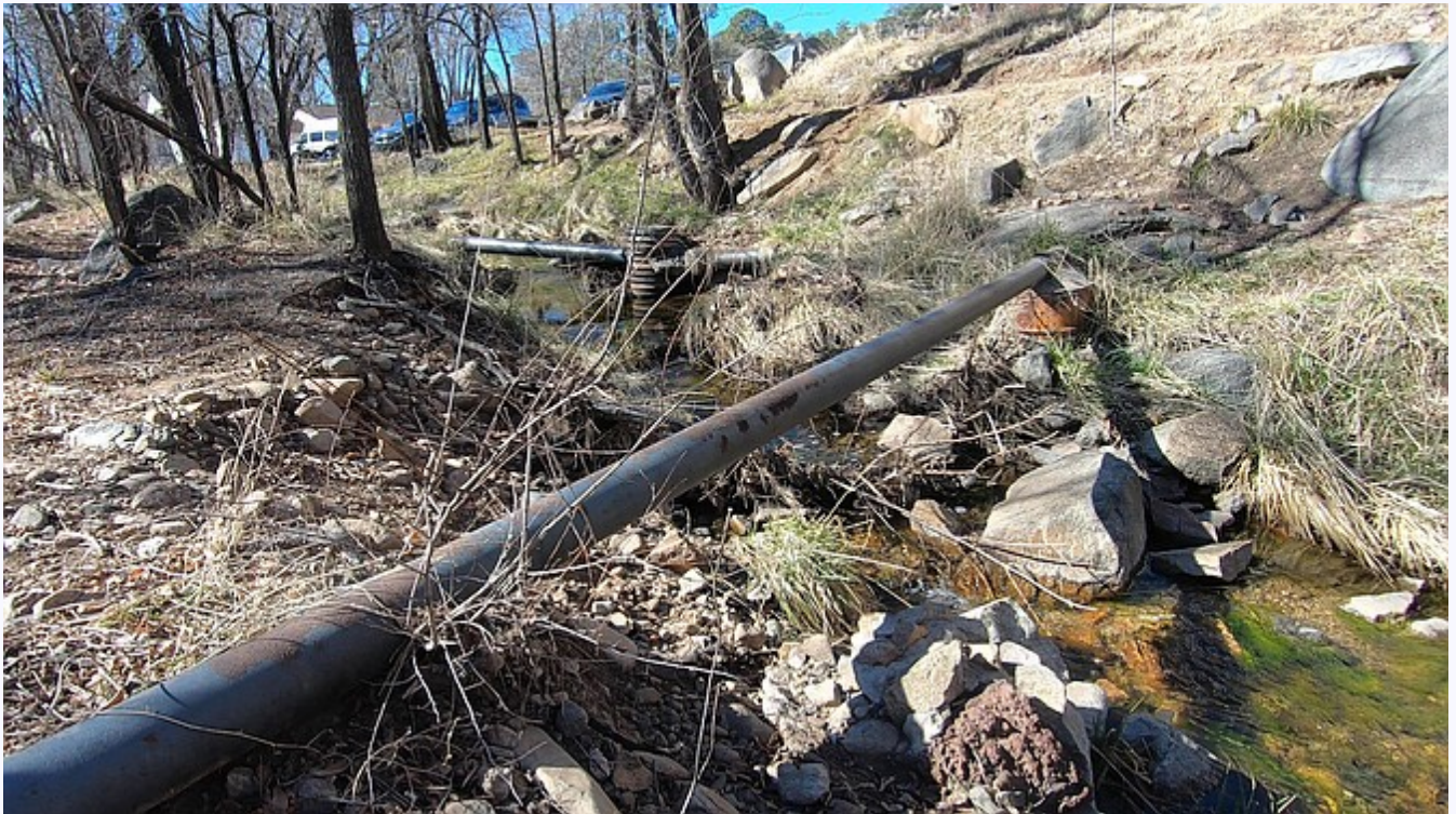
Outdated sewage lines cross Butte Creek on Friday, Feb. 7, 2020. (Jesse Bertel/Courier)
